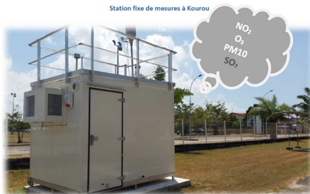
Figure 6 : Station de surveillance BRADY à Kourou, ORA 2017
