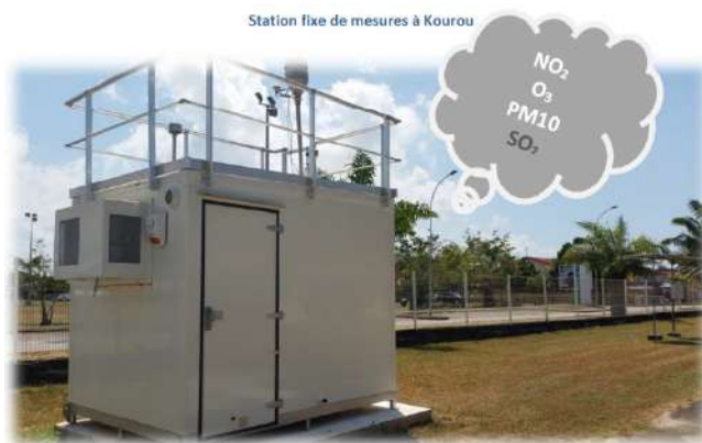
Figure 7 : Station de surveillance BRADY à Kourou, ORA 2017
