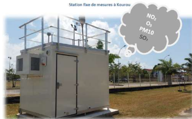
Figure 7 : Station de surveillance BRADY à Kourou, ORA 2017
